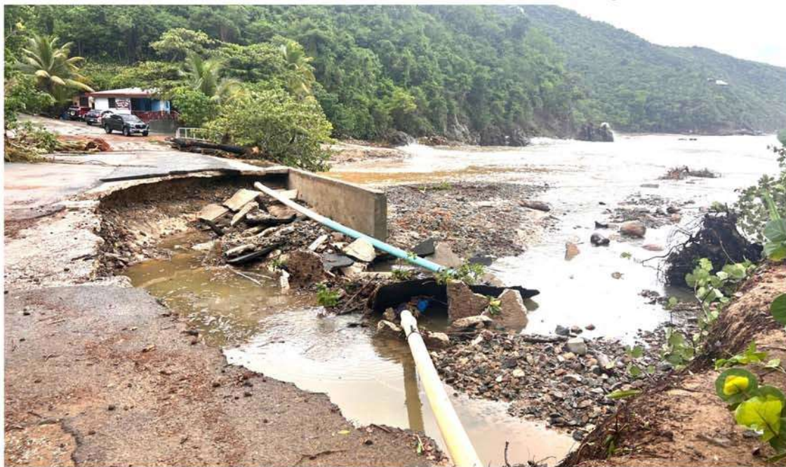
About 80 feet of the bridge in Brewers Bay was undermined when nine inches of rain fell from Tropical Storm Philippe, which left the underground water pipes exposed (Photo by Dean "The Sportsman" Greenaway)
