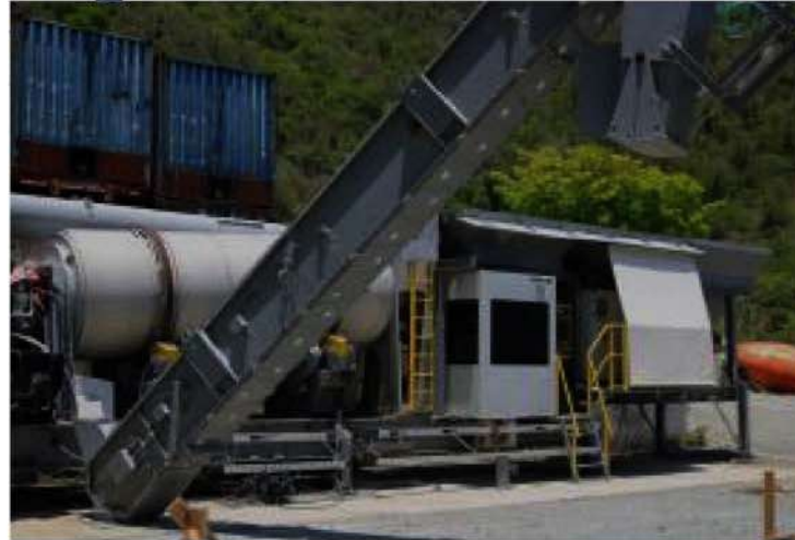
The Asphalt Plant
